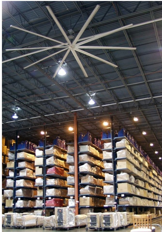
Figure 9. A large high-volume low-speed air circulating fan in a warehouse
