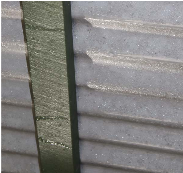
Figure 8. Condensation on underside of metal roofing
