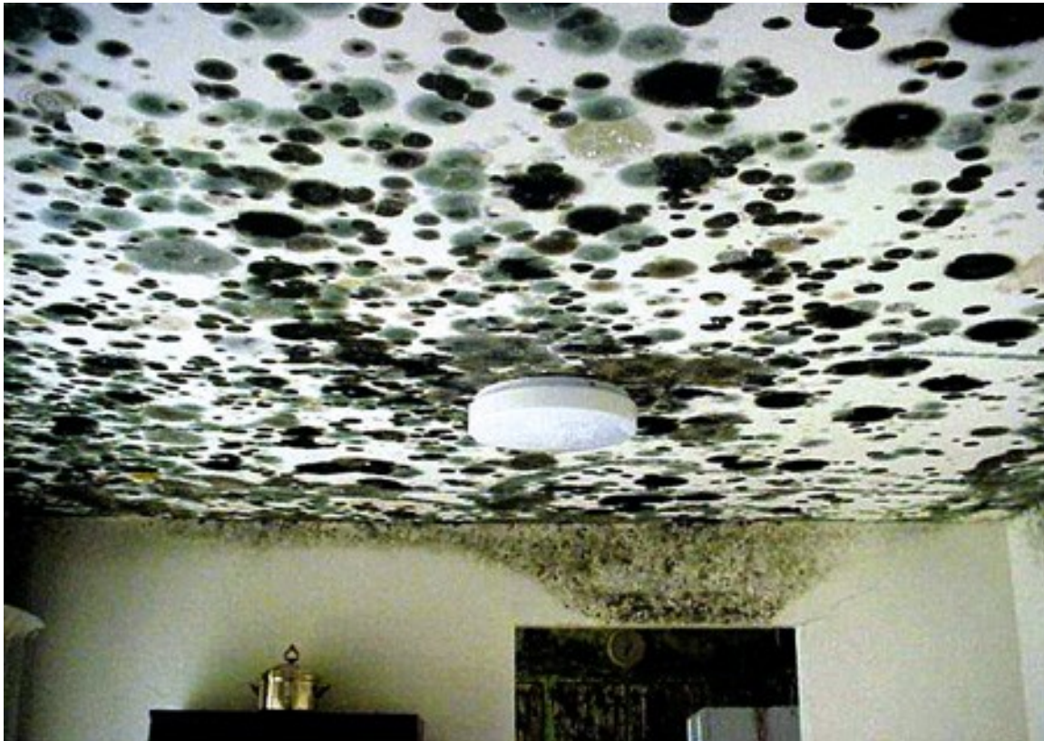
Figure 6. Mould on a ceiling due to moisture above
