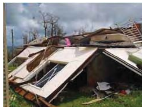
Photo 5 – inadequate tie-down through the entire structure
