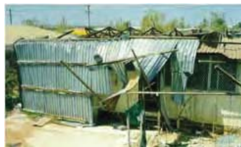
Photo 3 – inadequate batten to rafter connections (common in older housing)
