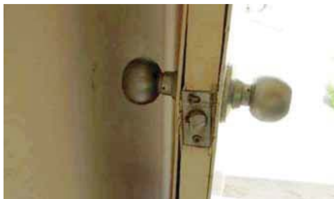
Photo 6 – Damage to door lock after high winds. Source: Cyclone Testing Station, James Cook University.
