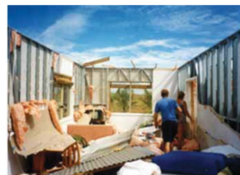
Photo 4 – inadequate roof truss anchorage
