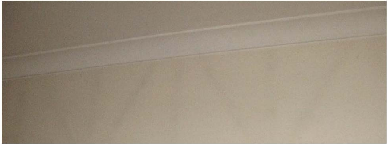
Figure 5.3 – Bridging of framing members combined with high indoor humidity can lead to patterned staining of plasterboard
