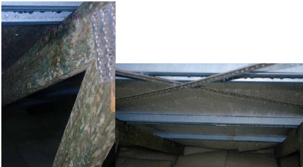
Figure A.8 Mould growth on roof trusses and condensation on the underside of the foil sarking
