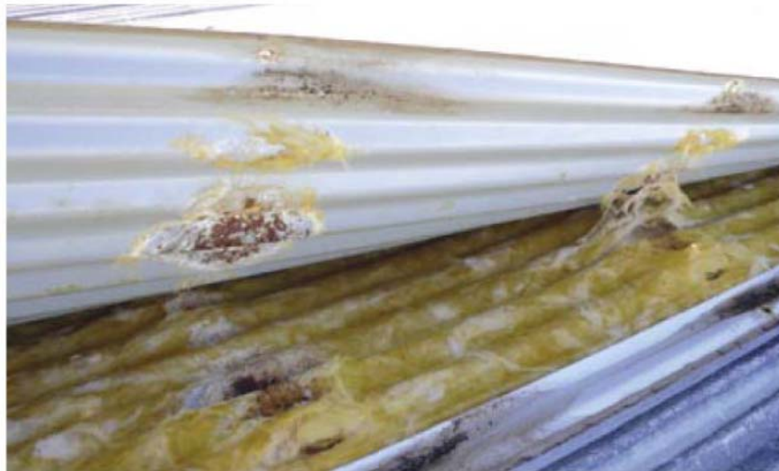
Figure 5.6 Photo showing moisture penetration due to the absence of a vapour barrier in a tropical environment
