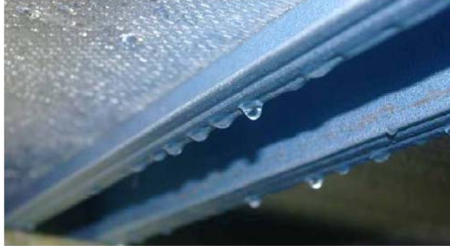
Figure A.7 Condensation on the impermeable foil sarking and purlins
