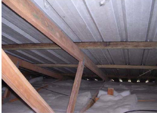
Figure A.6 Although the roof was ventilated by two wind driven ventilators at the eaves this was insufficient to prevent condensation.
